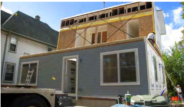
Top, Middle and Left Sequence showing the setting of a module for a house in Milwaukee.
